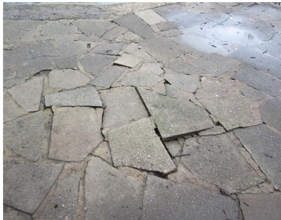
Hazardous crazy paving in need of repair
