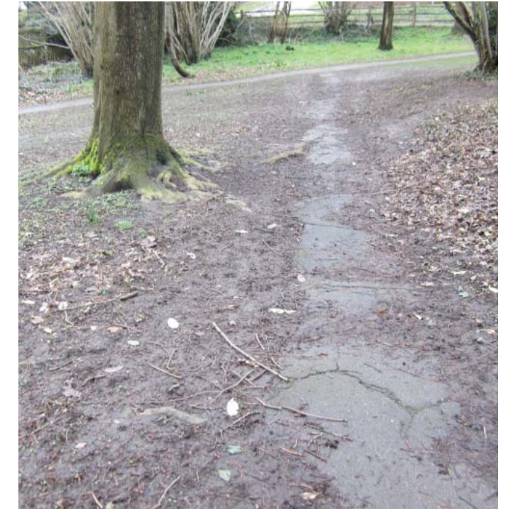
Macadam paths disintegrating
