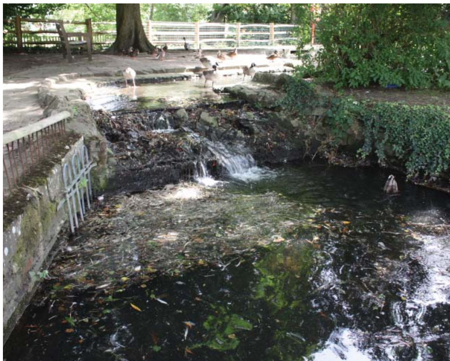
Waterfall wall in need of repair
