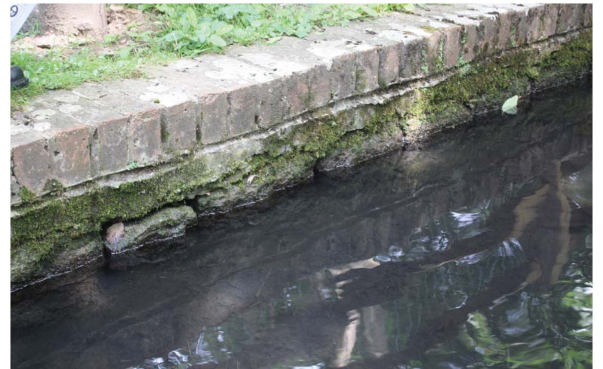
Repairs to stonework required
