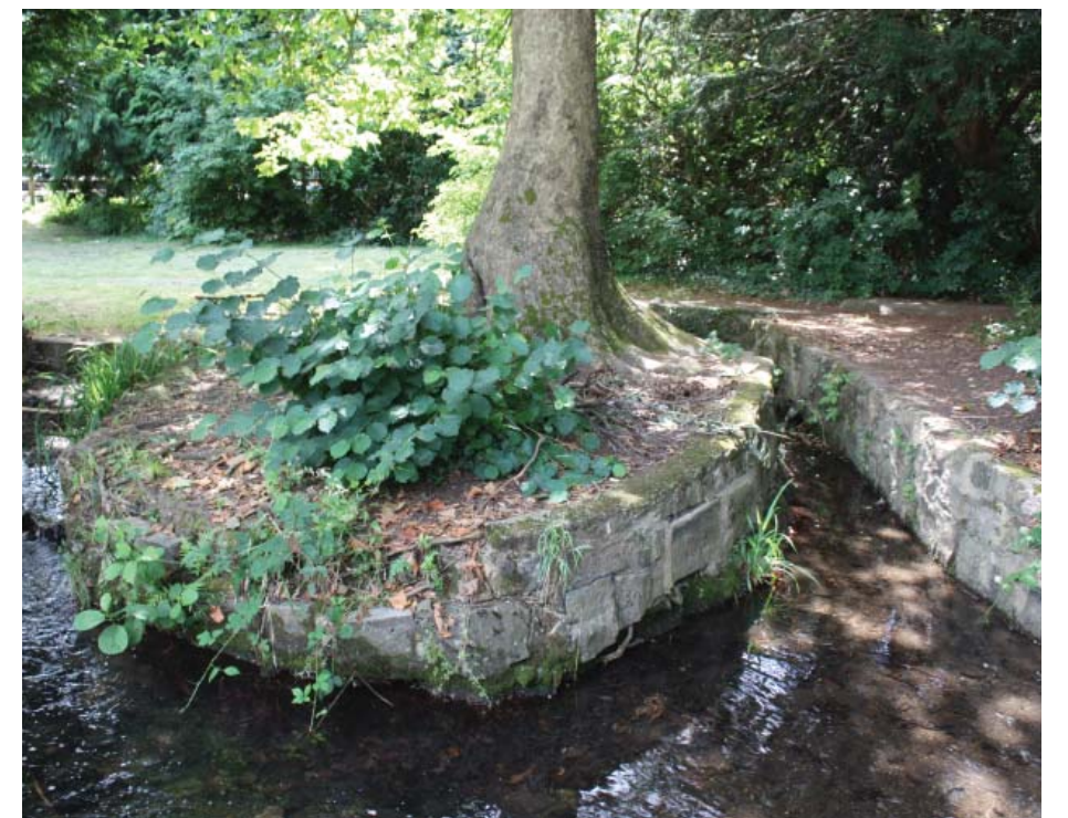
Tree roots pushing out stone walls
