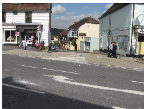
Photo 64 - HFS and road markings are worn
