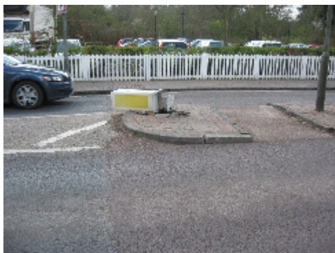
Photo 31 - Dislodged illuminating bollard
