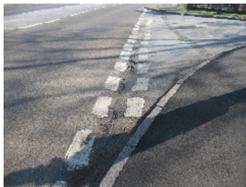
Photo 2 -Junction interface sunken and breaking up
