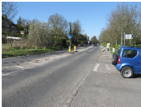
Photo 12 - Flecta Bollards coated in grime
