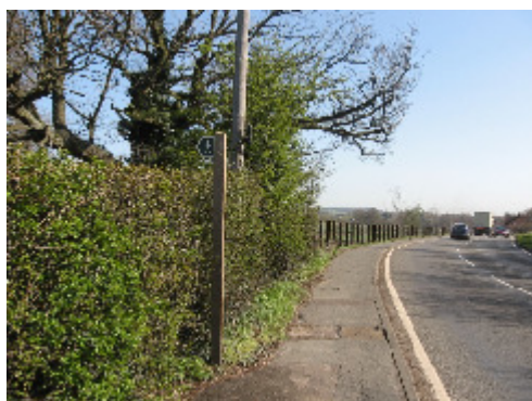
Photo 47 - Footpath broken away at 'Post Office Telephones' utility cover
