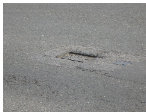
Photo 16 - Road surface is deteriorating
