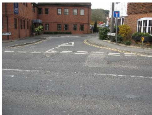
Photo 70 - Carriageway has sunken and junction mouth deteriorating
