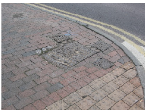
Photo 36 - Sunken utility covers
