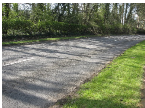
Photo 55 - Carriageway is deteriorating
