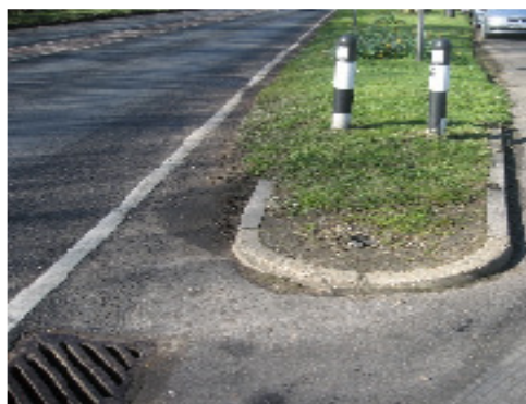
Photo 6 - Road marker post missing
