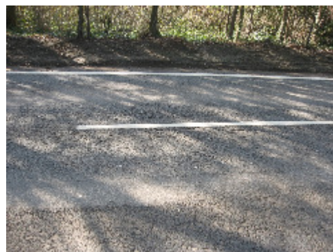
Photo 43 - Road surface deteriorating
