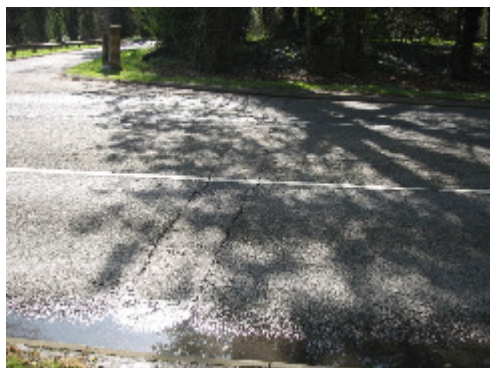
Photo 49 - Rutting in the carriageway
