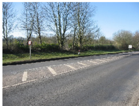
Photo 5 - Road marker posts have been dislodged and the repeater sign is coated with grime
