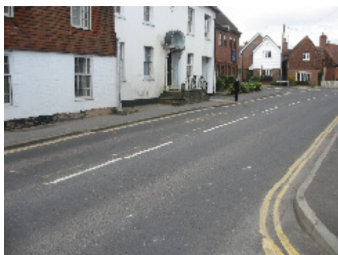
Photo 71 - Bus road markings are worn
