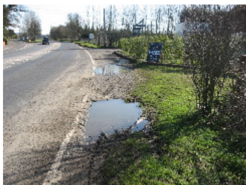
Photo 10 - Lay-by is in a poor
