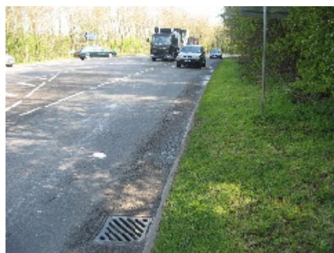
Photo 52 - Carriageway edge is deteriorating
