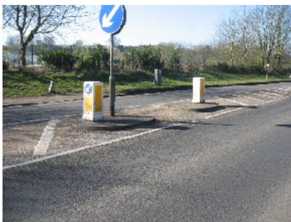
Photo 3 - A feeder pillar is dislodged and the illuminated bollards coated in grime
