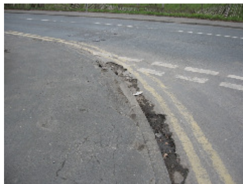
Photo 23 - Junction interface deteriorating
