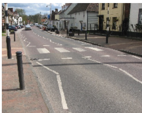
Photo 33 - Road markings are worn
