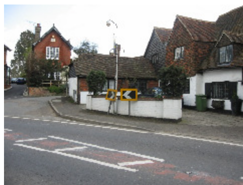
Photo 72 - Chevron signs are coated in grime and one has been dislodged
