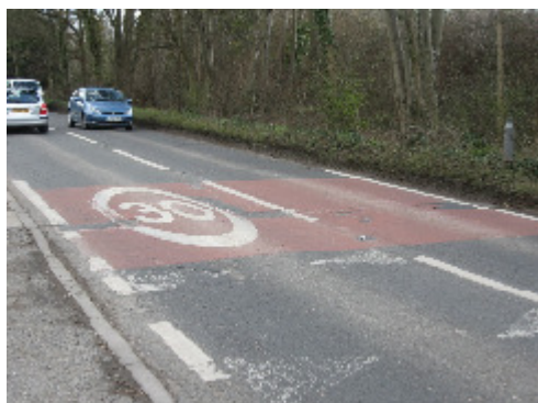
Photo 42- HFS broken away and road markings are worn
