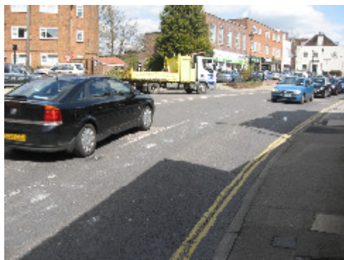
Photo 69 - Carriageway centre line is worn
