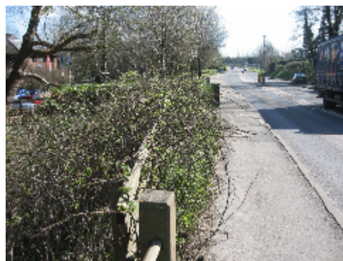
Photo 14 - Thorny vegetation encroaching onto footpath
