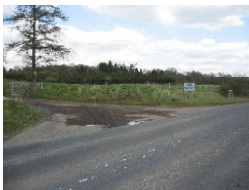
Photo 79 - Junction mouth is in a poor condition
