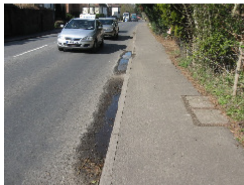
Photo 20 - Ponding on carriageway
