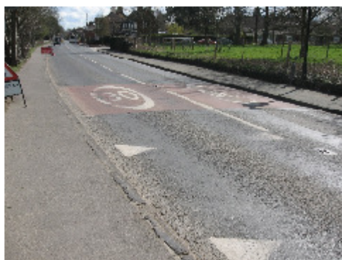
Photo 24 - Road markings are worn
