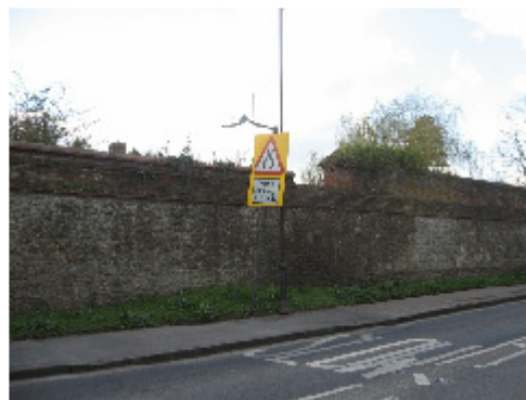
Photo 28 - Dislodged sign and worn 'Slow' road marking
