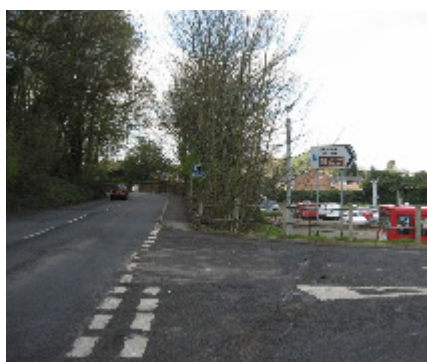
Photo 59 - Junction mouth deteriorating
