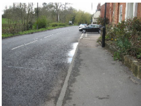
Photo 73 - Ponding in carriageway
