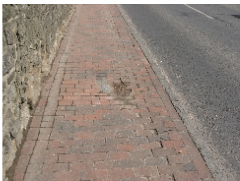
Photo 34 - Footpath has sunken
