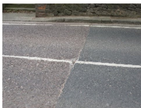
Photo 39 - Pothole in carriageway
