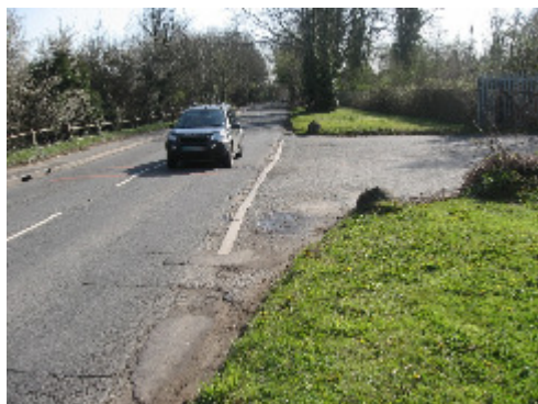
Photo 44 - Junction interface is in a poor condition
