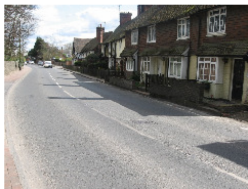
Photo 37 - Road markings are worn
