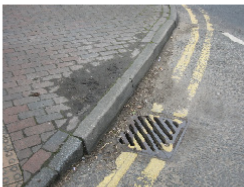
Photo 29 - Yellow lines are worn and gully is blocked
