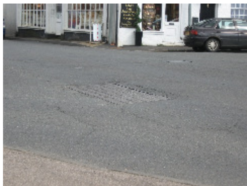
Photo 17 - Road surface is deteriorating
