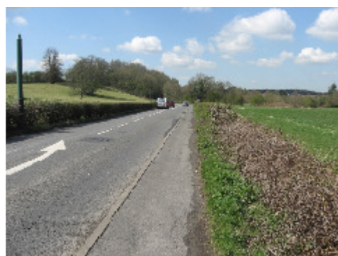
Photo 56 - Footpath verge subsiding
