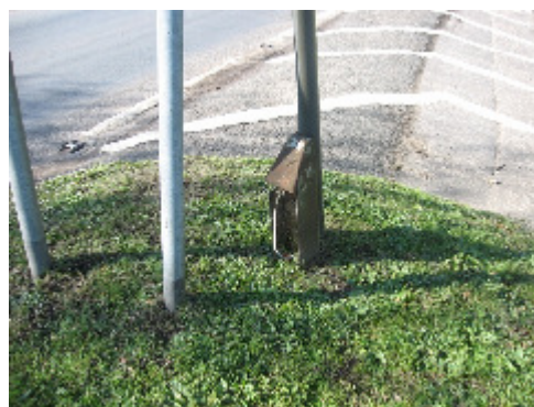
Photo 9 - The panel cover is missing
