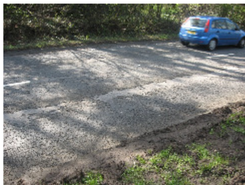
Photo 53 - Road surface is deteriorating
