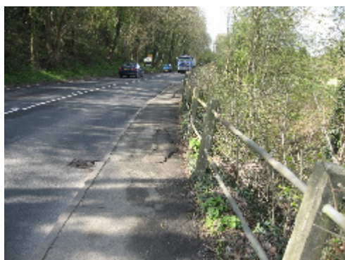
Photo 57 - Footpath is subsiding
