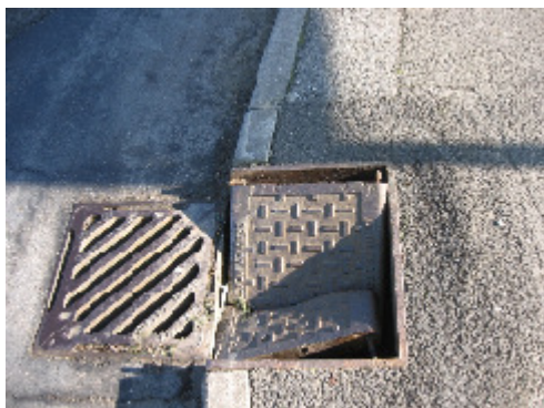
Photo 1 - Kerb entry gully cover broken
