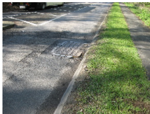
Photo 50 - Manhole cover surrounds breaking up
