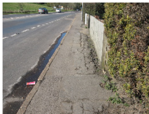
Photo 7 - The footpath is deteriorating
