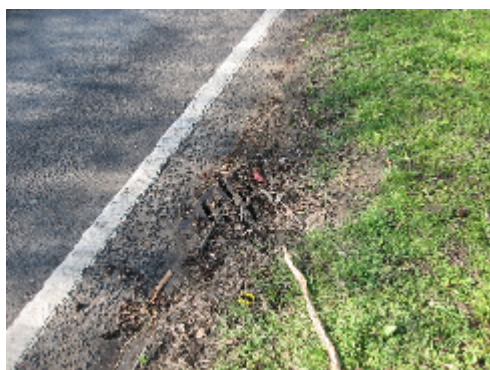
Photo 8 - Gullies are blocked
