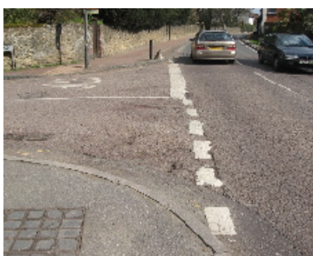
Photo 38 - Junction mouth is in a poor condition
