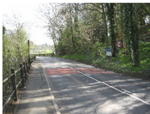
Photo 58 - HFS is breaking up and worn
