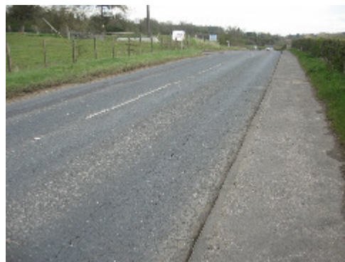
Photo 78 - Carriageway cracking and evidence of deterioration
