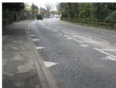
Photo 26 - Footpath is deteriorating
